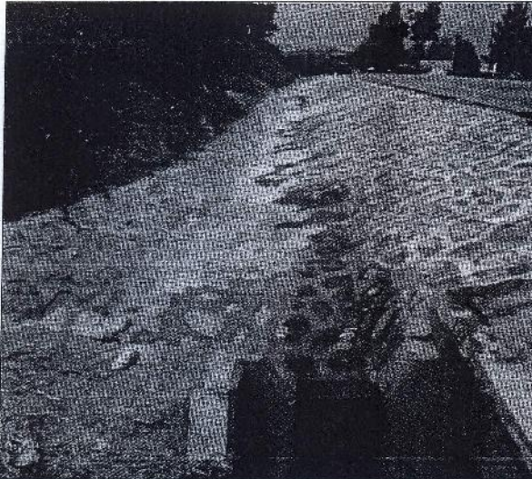
Km 41+110 to km 41+257 LHS; repair of stone pitching at culvert drop-inlet and ditch lining
